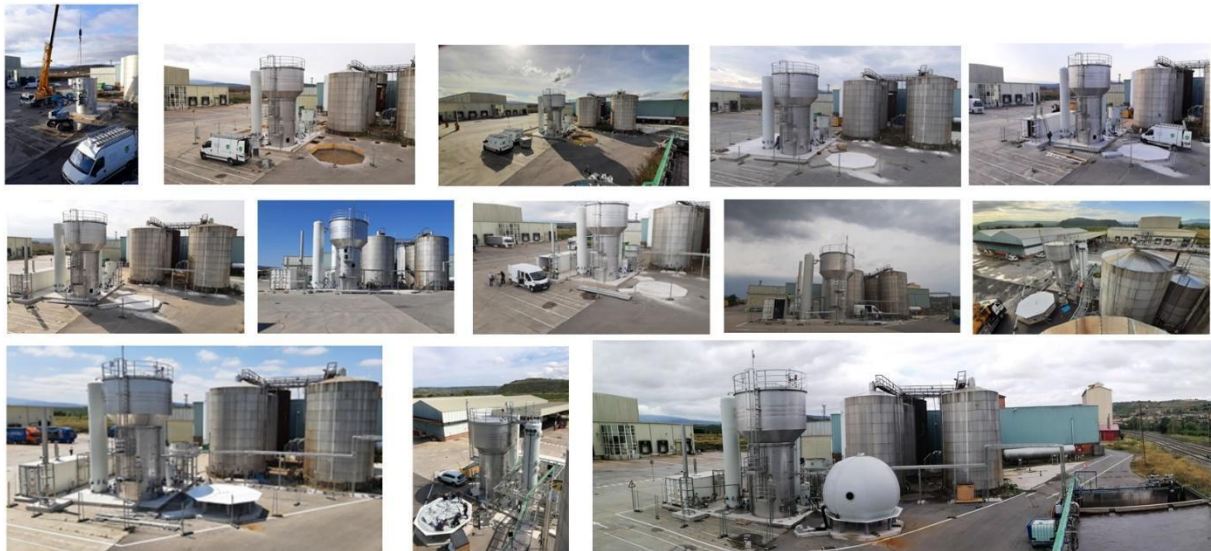
Figure 22. Civil work equipment installation, as well as mechanical and electrical assembly in AGE Winery (Fuenmayor, SPAIN) to build the LIFE Multi-AD demo unit.
