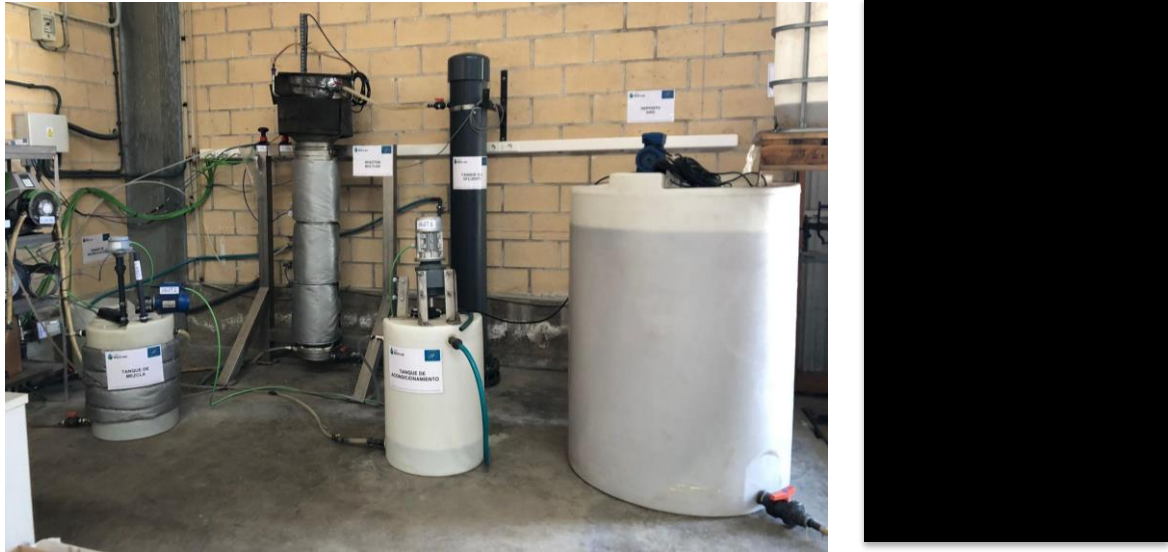
Figure 36. 100 L LIFE Multi-AD technological solution installed at AEMA (Alfaro) and anaerobic reactor dimension.
